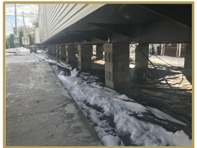
Flood resistant foundation with tie-down straps
